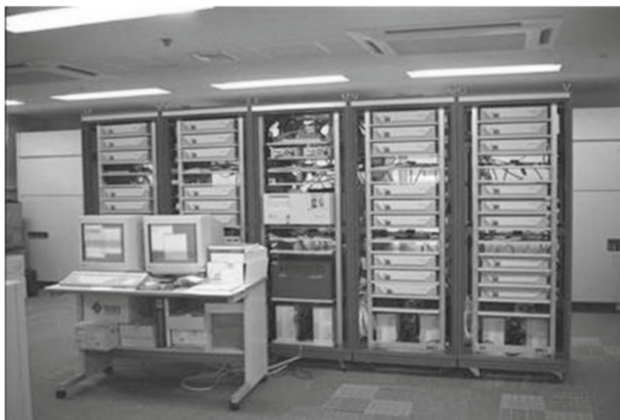
Fig. 8.1 Workstation cluster of 36 Sun workstations connected with Myrinet installed at RWCP, 1996. This cluster was used to develop the first version of SCore
